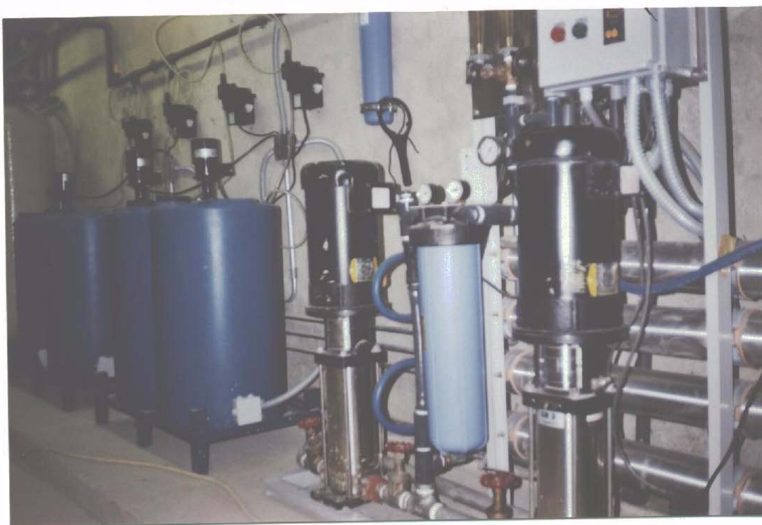
Reverse Osmosis plant, Gandour Villa Chamlan , Lebanon .
