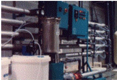
35,000 gpd System With Level Control and Pump Controls
